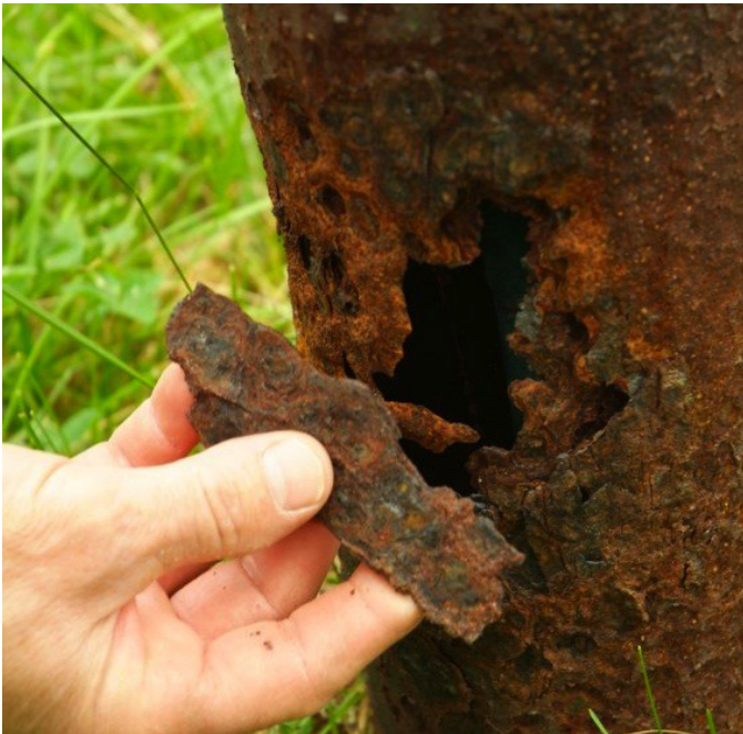
Hole in casing caused by corrosion.
