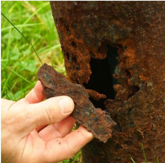
Hole in casing caused by corrosion.
