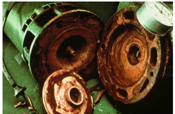
Abrasion caused by pumping sand.
