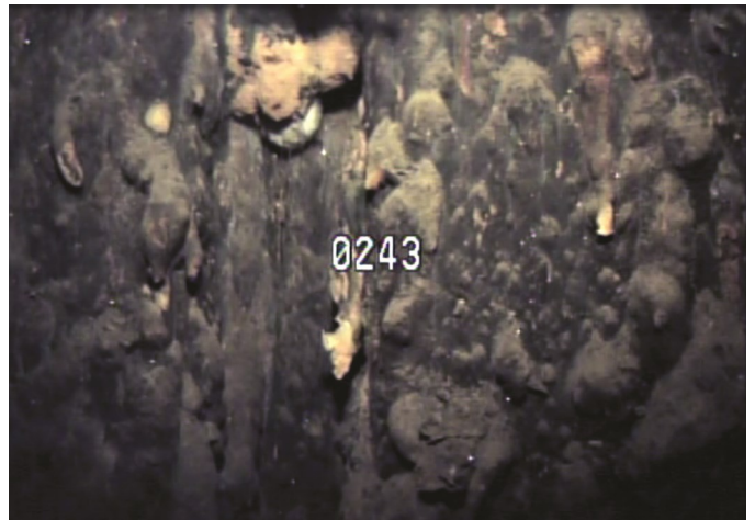
Well video image showing heavy biological and scale fouling, completely covering the screened section of the well.
